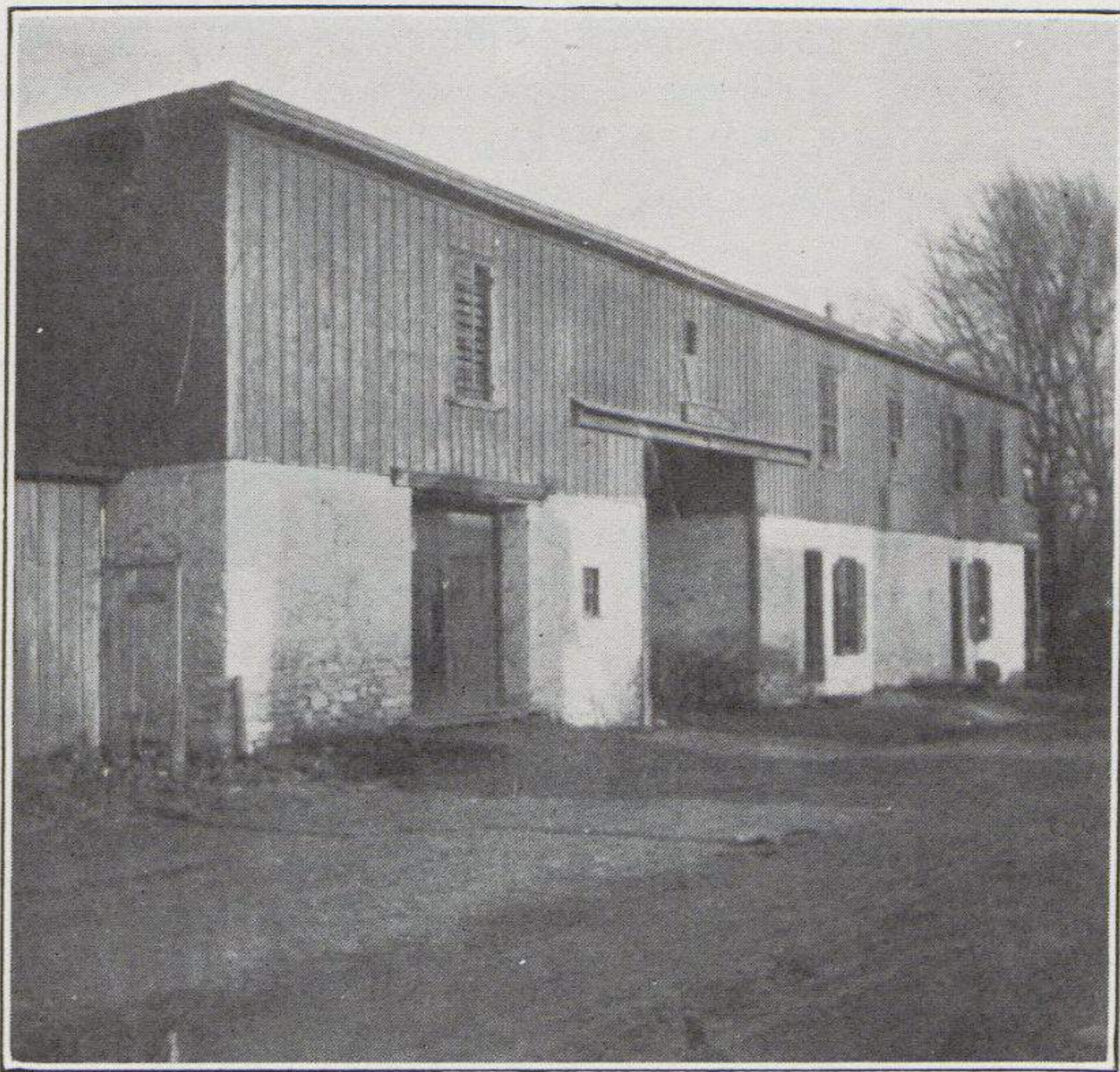
FORMER STABLE—BRYN MAWR. NOW A TENEMENT. NINE PERSONS SLEEP IN ONE ROOM—FRANKLY IMMORAL CONDITIONS.
